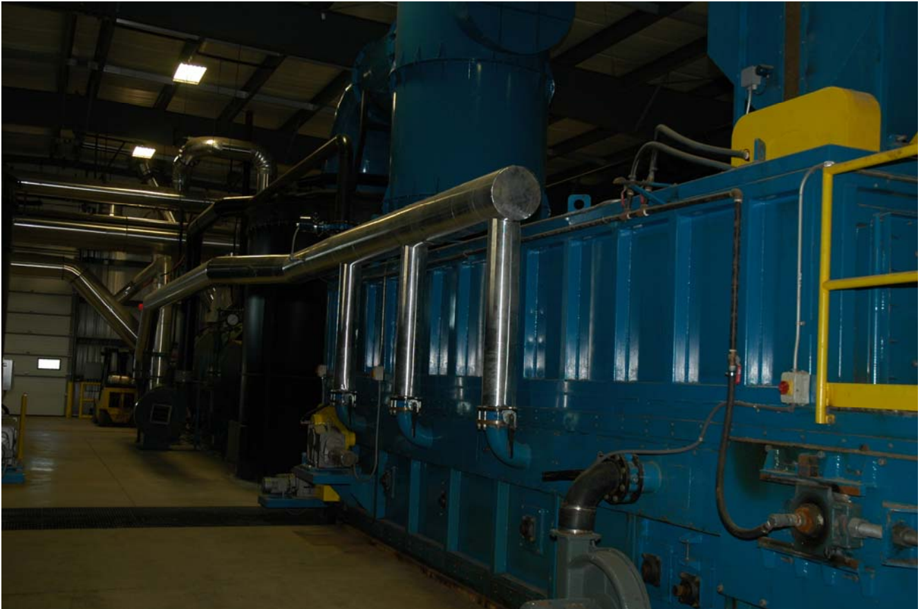
Figure 2 Gasifier System looking towards Boiler
